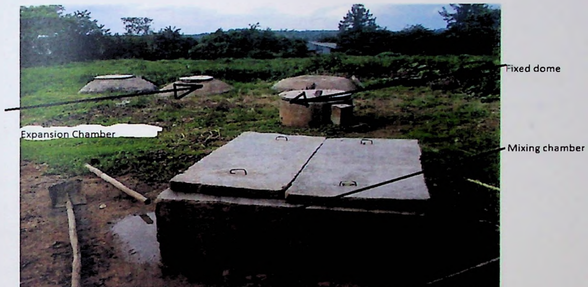
Figure 4.1: Fixed dome digester installation
