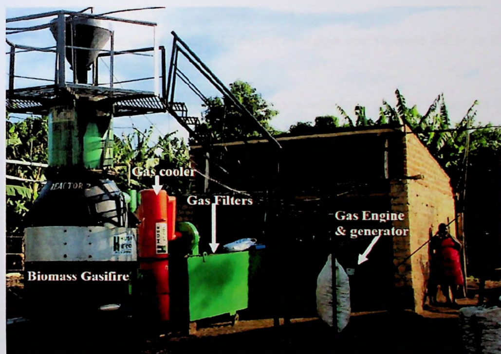
Figure 3.2: A pilot HPS installed at Tiribogo village, Muduma sub-county, Mpigi District (1st HPS in Uganda)
